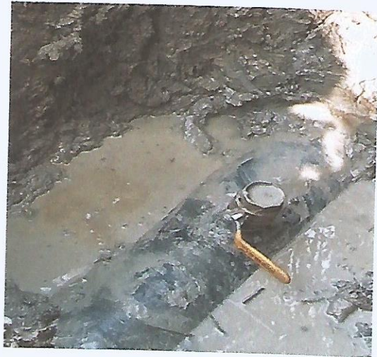
Fig 2. Showing theft point after excavation.
